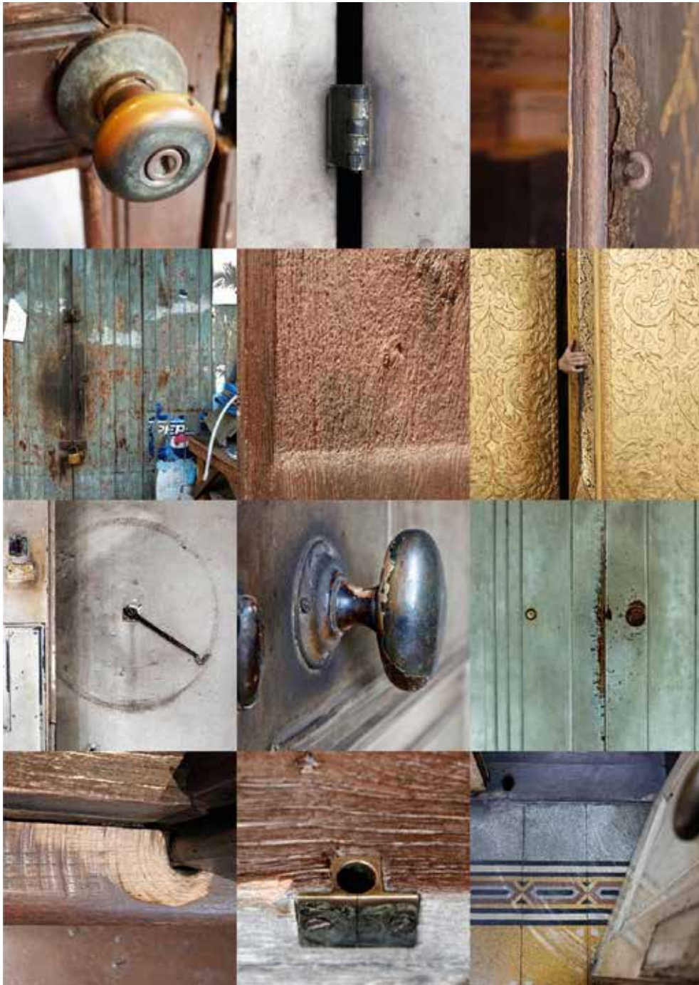
Figure 1: Opening doors and crossing thresholds. Observing old, well-preserved, perfectly neglected architecture, the patterns of wear from both intended and incidental use are conspicuous. The sun, the rains, hands, and movements all leave their marks. Source: author .
